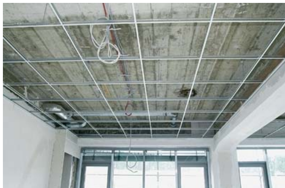
Ceiling with first line of hangers set at less than half the normal span from each edge
