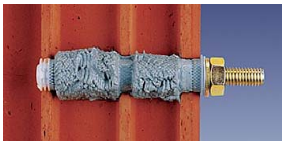
A threaded rod set in a hollow clay pot using injection resin and a perforated plastic sleeve
